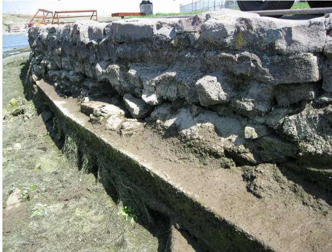
Photo Showing Condition of Existing Wall, Fishing Stations Shown in Upper Right Photo Taken August 24, 2009 During Drawdown of Rainbow Reservoir
