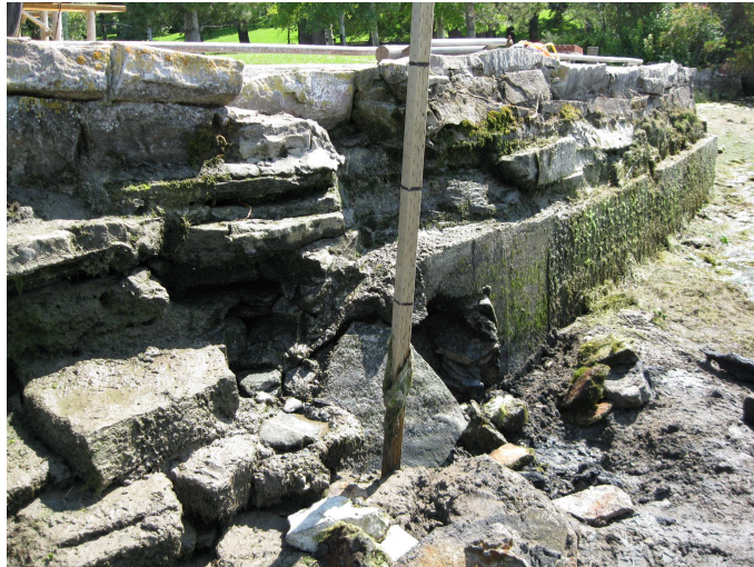
Photo Showing Condition of Existing Wall Photo Taken August 24, 2009 During Drawdown of Rainbow Reservoir
