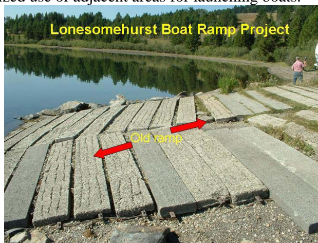
Old ramp is too steep, gaps are unsafe, and rip-rap is not functioning
