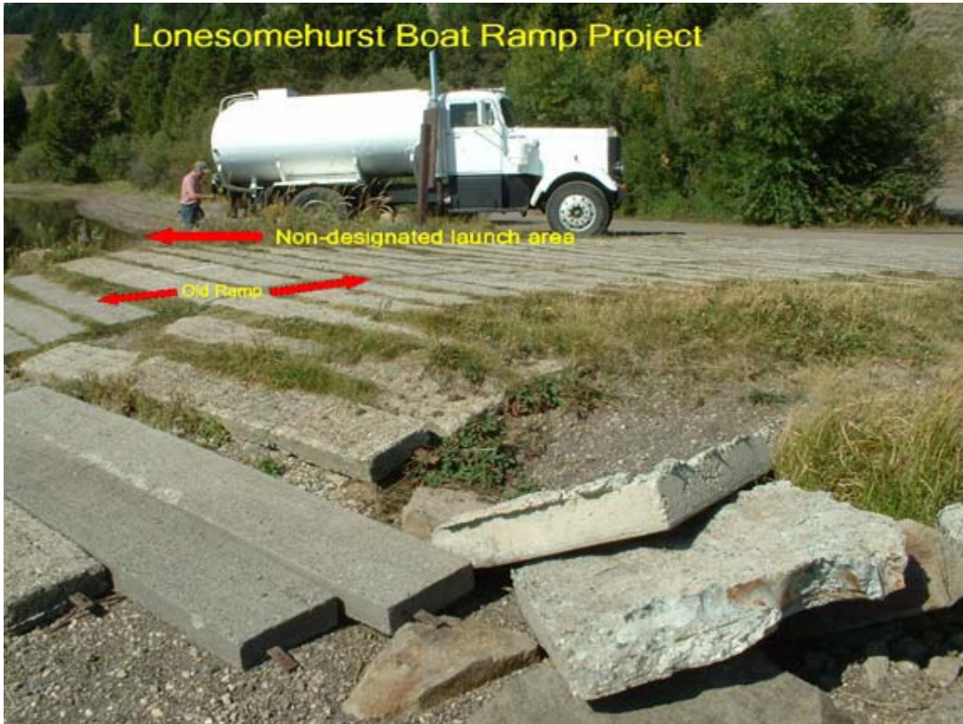
Old ramp is unsafe and unsightly. Users have created there own launch (upper left)
