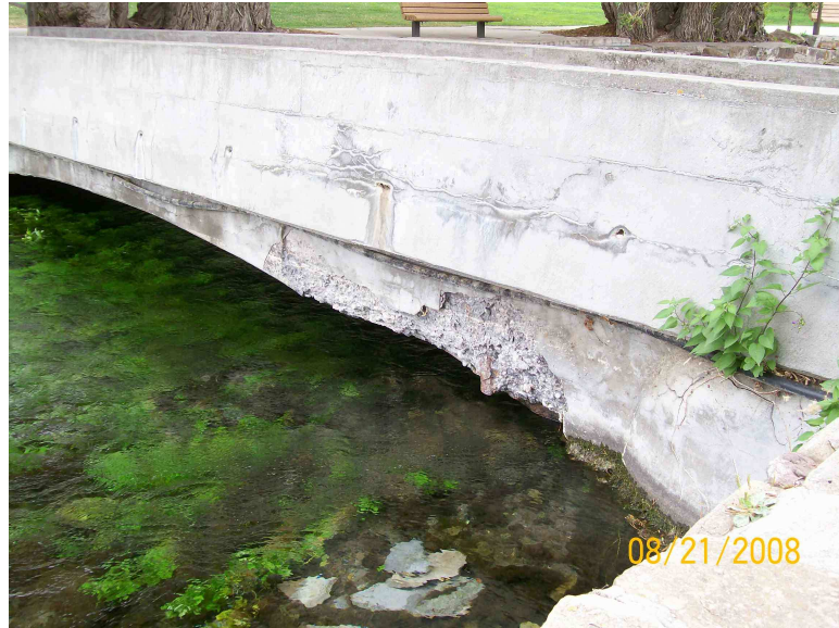
Photo Showing Spalling of Roe River Bridge – North Side
