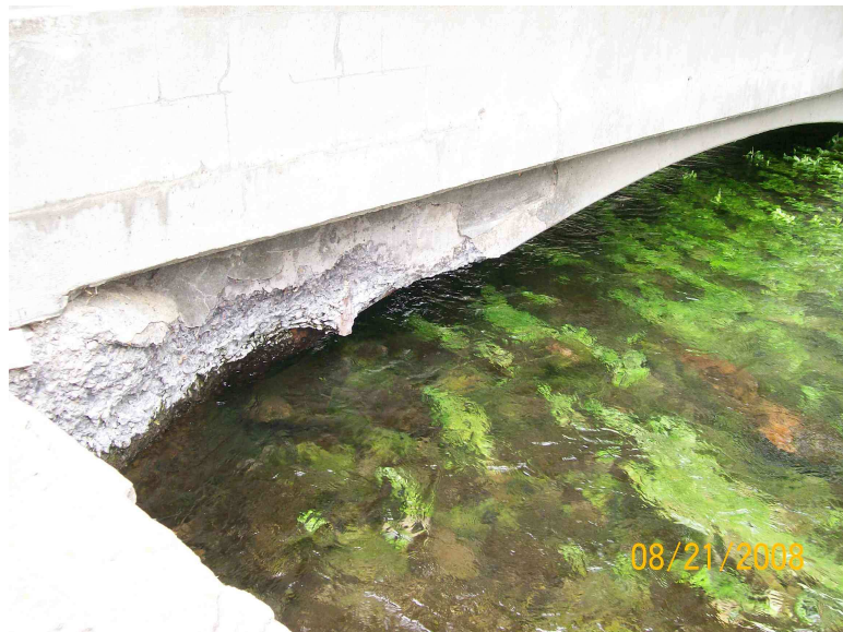
Photo Showing Spalling of Roe River Bridge – South Side
